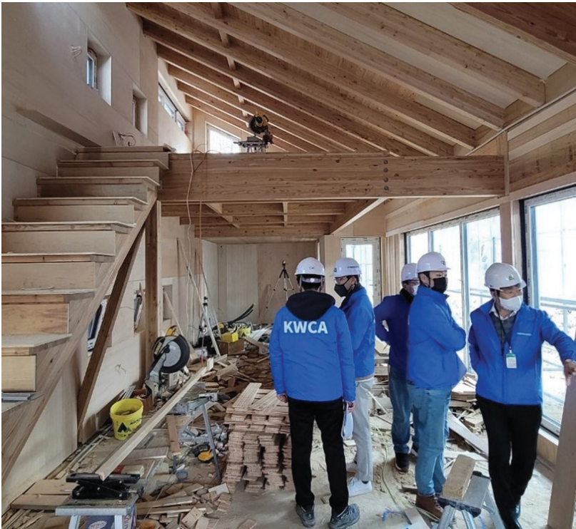
KWCA's 5-star inspectors at the site of Gaho-dong Annex Building | Photo: Korea Wood Construction Association
