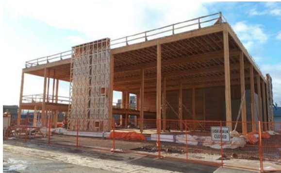
Figure 1. Wood Innovation Research Lab glulam post and beam structural system with vertical truss wall panel to be insulated on site.
