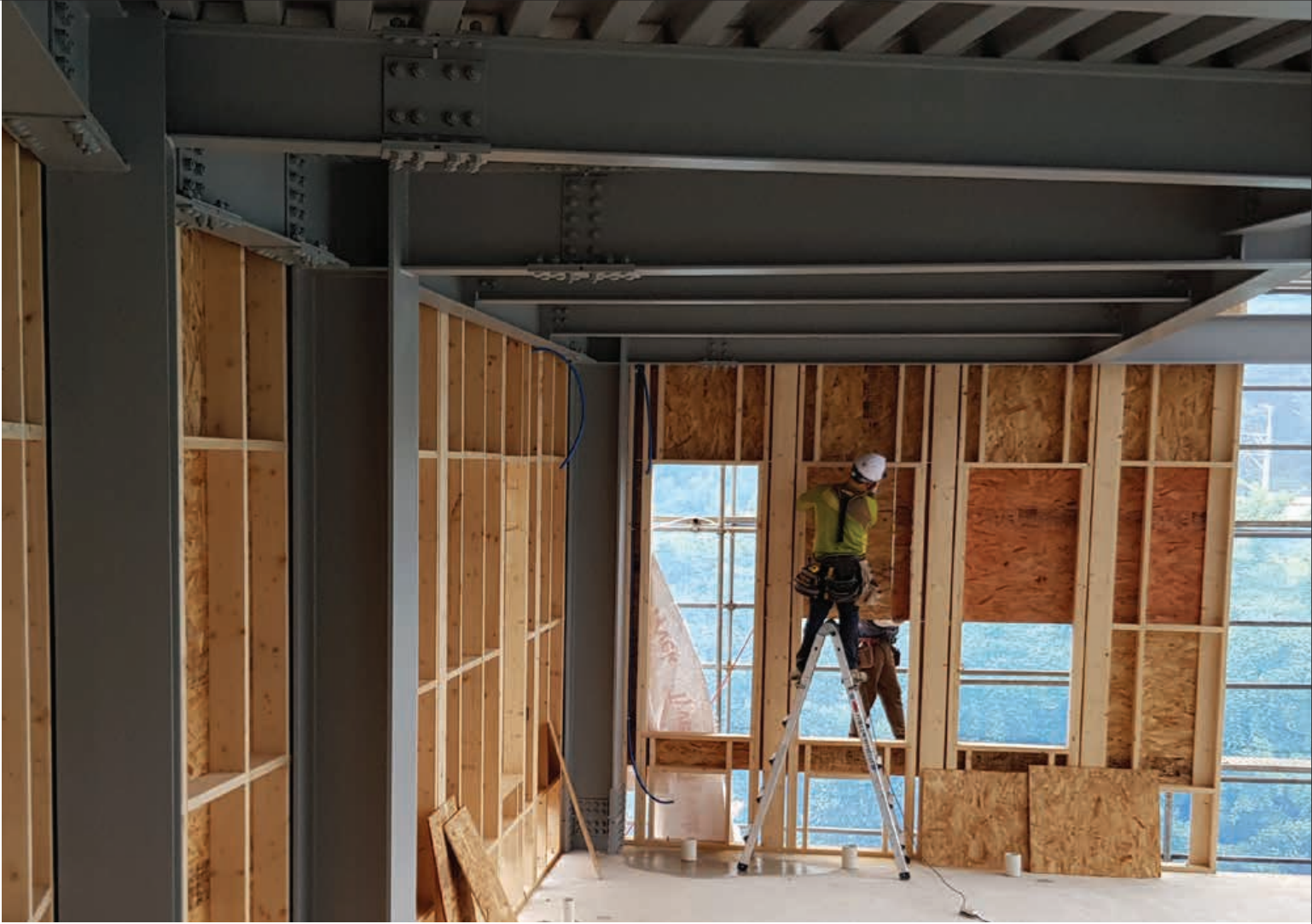
Cheongpyeong Cultural Centre steel and wood infill wall project, Gyeonggi province | Photo: Canada Wood Korea
