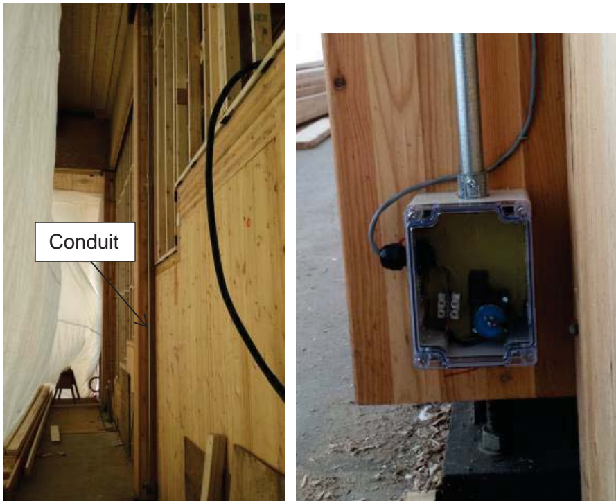
Figure 2 A displacement sensor (its metal conduit in left photo, and a closer image of the sensor box which is just above the column base metal connector) at Location 1 for measuring vertical movement of the glulam column
