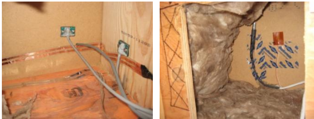
Figure 7 Photo of two installed MC pins and one moisture detection tape (left, on MDF sheathing and a stud) and an RH/T sensor and a heat flux sensor (right, interior of MDF sheathing)
